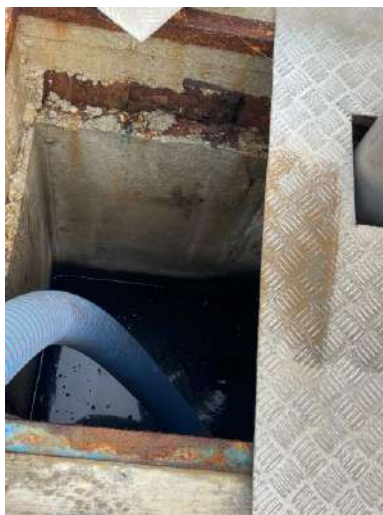
Figure 5 (c): Water Draining from the laundry
